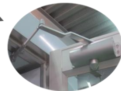
Door Closer Installed from inside
